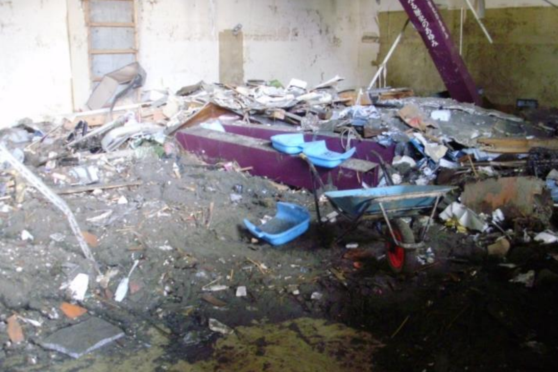
First Floor Exhibition Room after debris removal: more than 1m of sand accumulated on the floor
